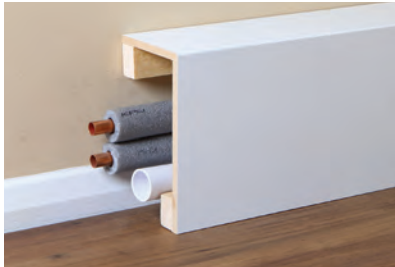
Pipe & Fire Sprinkler Boxings
