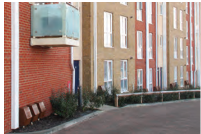
Metal Pipe Boxings
