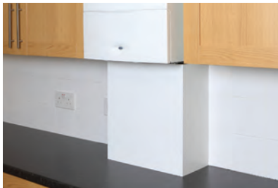
Boiler Pipe Boxings
